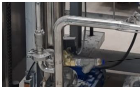
Water inlet of Condenser, DN20
