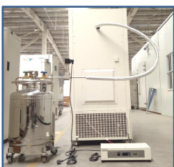
LN 2 /CO 2 backup system
